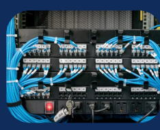
CABLING , DRESSING & LABELING
